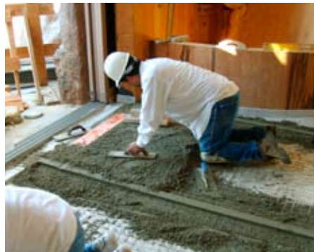
Like natural stone, a thick set mortar bed can be used when installing large format tile.
