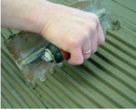
A medium-bed (thin-set) method, utilizing large trowel sizes and mortar with anti-slump characteristics, is most common when installing large format tile.
