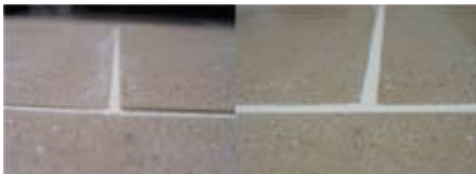
Large format tile set in a staggered pattern can exacerbate lippage that is more obvious with narrow grout joints.
