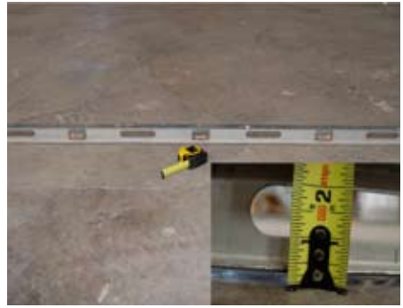
Although, the TCA Handbook calls for 1/4-inch maximum deviation from planarity every 10 feet, one should consider even stricter tolerances when working with large format tile
